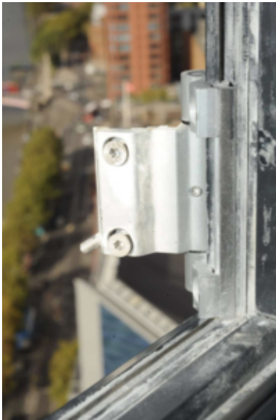
Close up of window frame and bracket taken by police in Oct 2018
