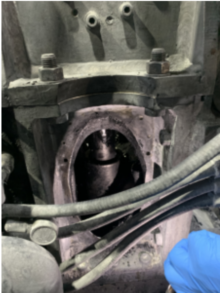
Close up of the hydraulic ram
