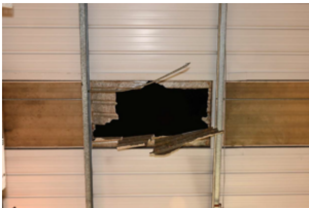
Broken roof skylight
