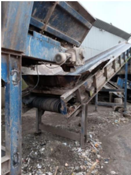
The unguarded conveyor
