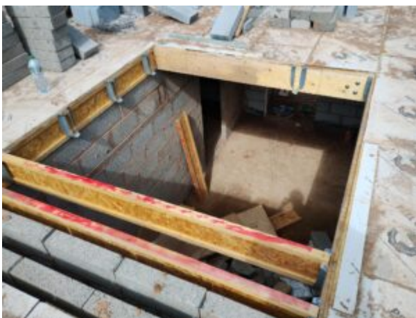
The collapsed stairwell after the incident
