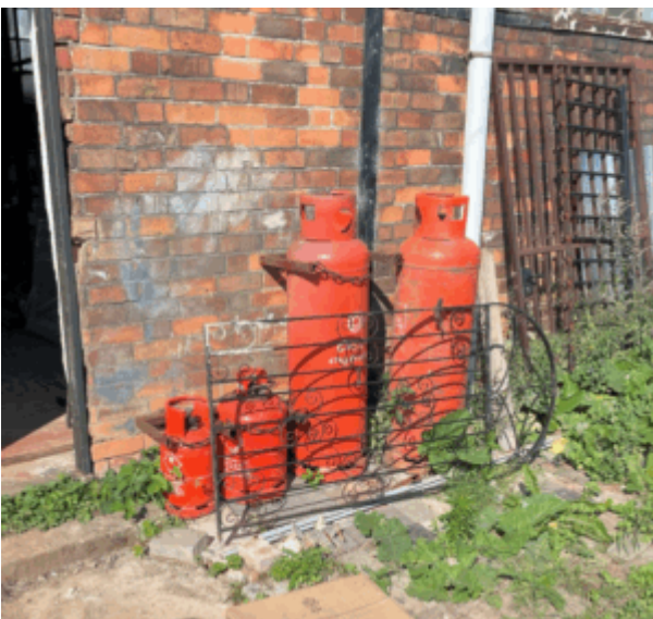
Unsafe storage of flammable gas
