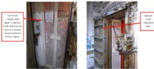
Figure 11 – Lift Entrance and Watertight Door in P-M-12
