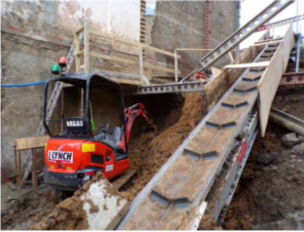
excavation and stability structure concerns
