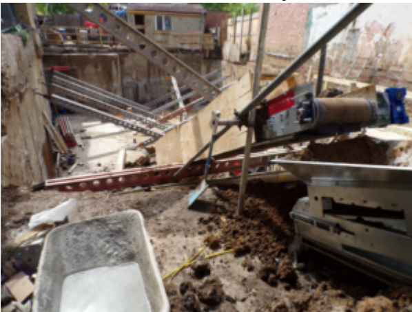
work at height fall risk from open edge
