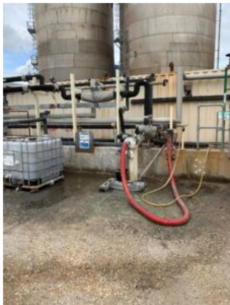
The Caustic Loading area from the ICL site
