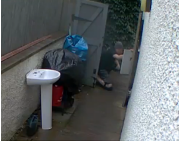
Lee Lancaster carrying out illegal gas work
