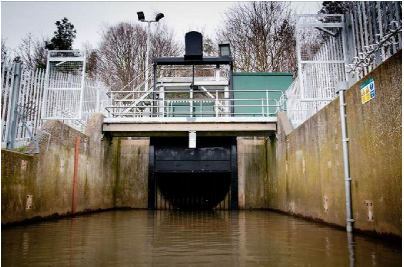
The lifting screen at Primrose Hill
