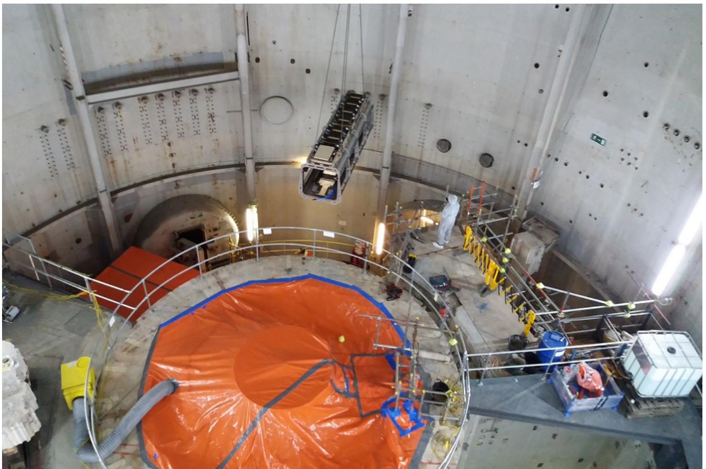
LaserSnake and its housing are lifted into place at the Dragon reactor
