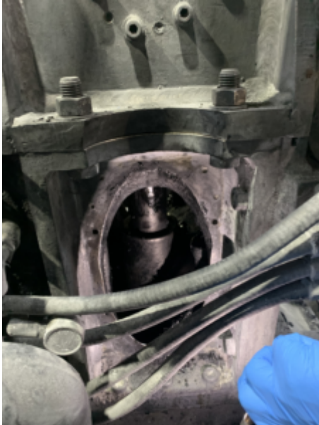
Close up of the hydraulic ram
