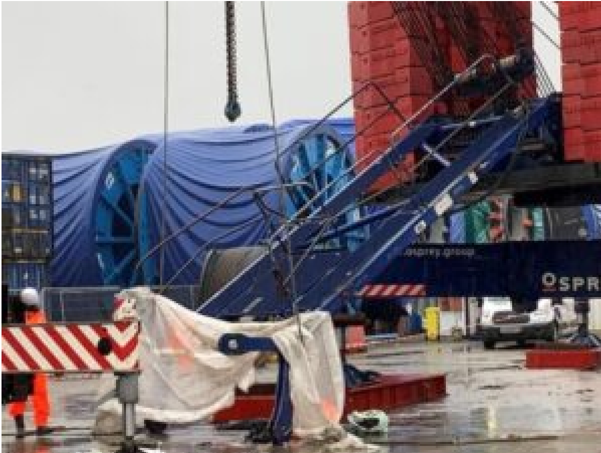
The collapsed platform
