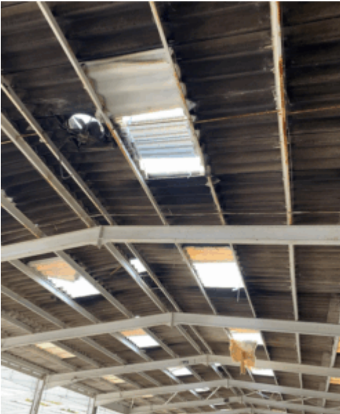
the worker fell from this roof
