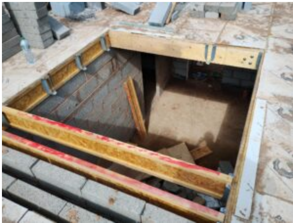
The collapsed stairwell after the incident
