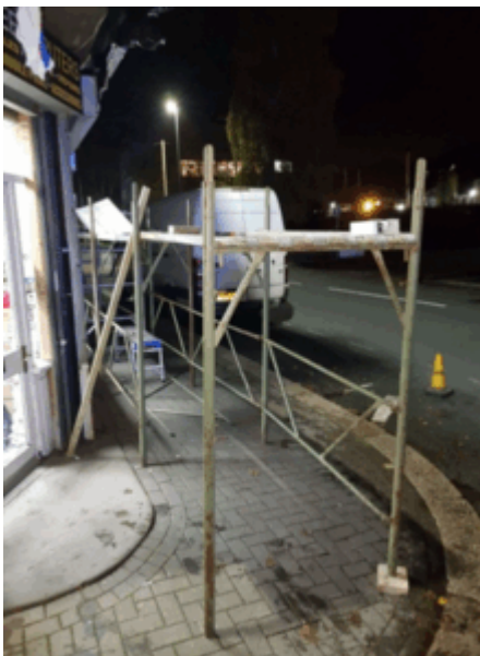
The scaffolding tower without edge protection
