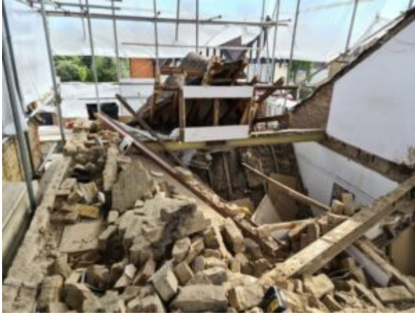
The devastation following the collapse
