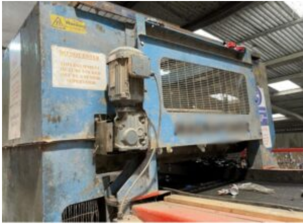
Waste sorting line machinery
