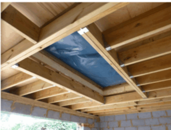
Tarp covering roof/hole when HSE attended
