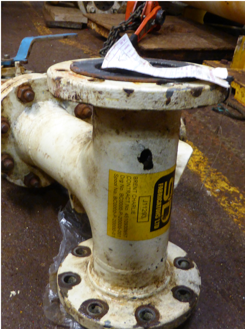
Spool with the corrosion failure identified.
