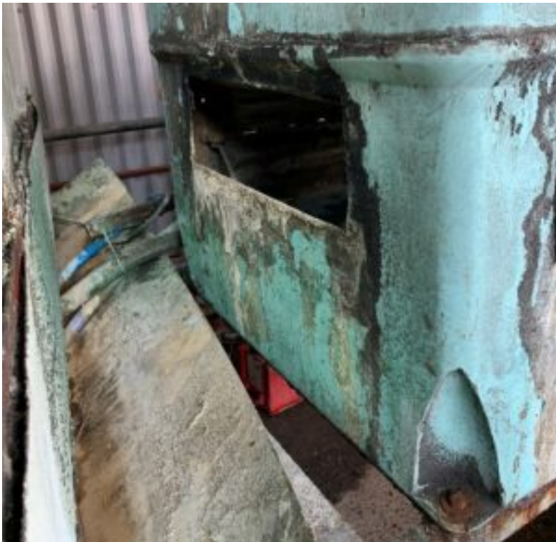
One of the water-cooling towers at Riaar Plastics Limited
