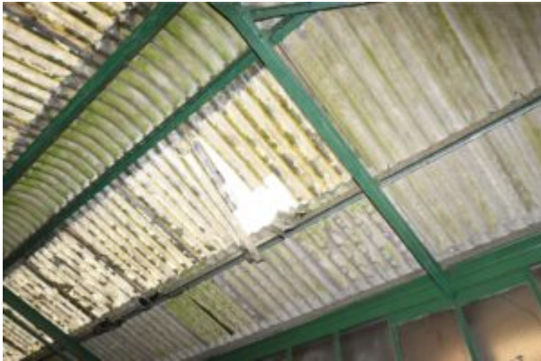
The hole left in the roof
