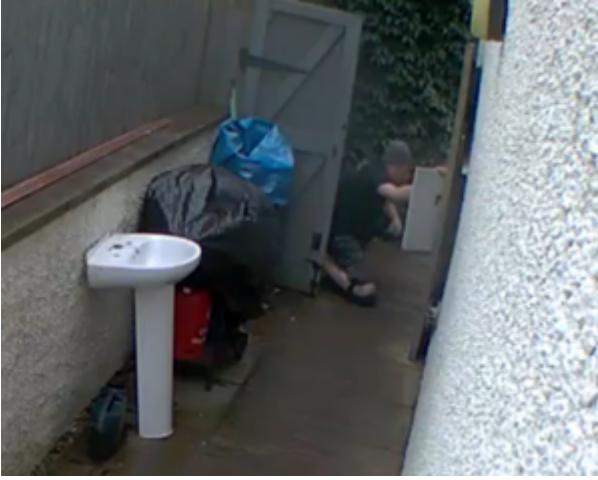
Lee Lancaster carrying out illegal gas work
