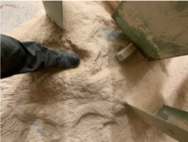
An inspector's boot shows the scale of the wood dust found
