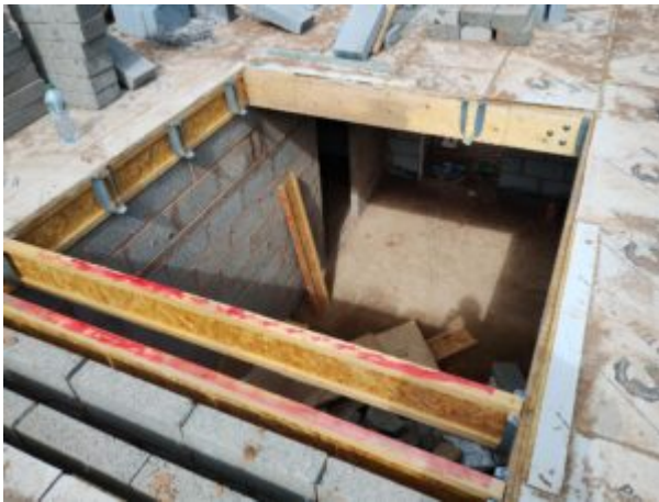
The collapsed stairwell after the incident
