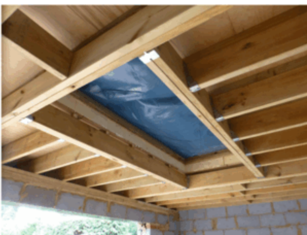
Tarp covering roof/hole when HSE attended
