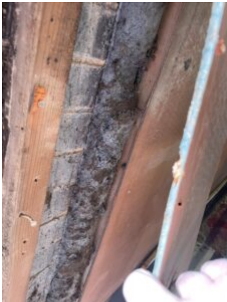
Section of the removed wall panelling containing asbestos
