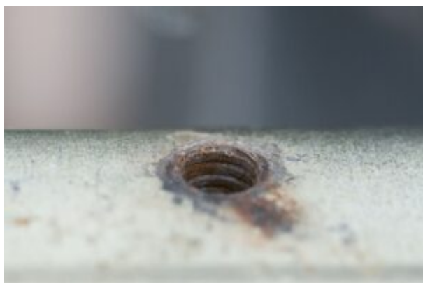
One of the bolt holes on the guard
