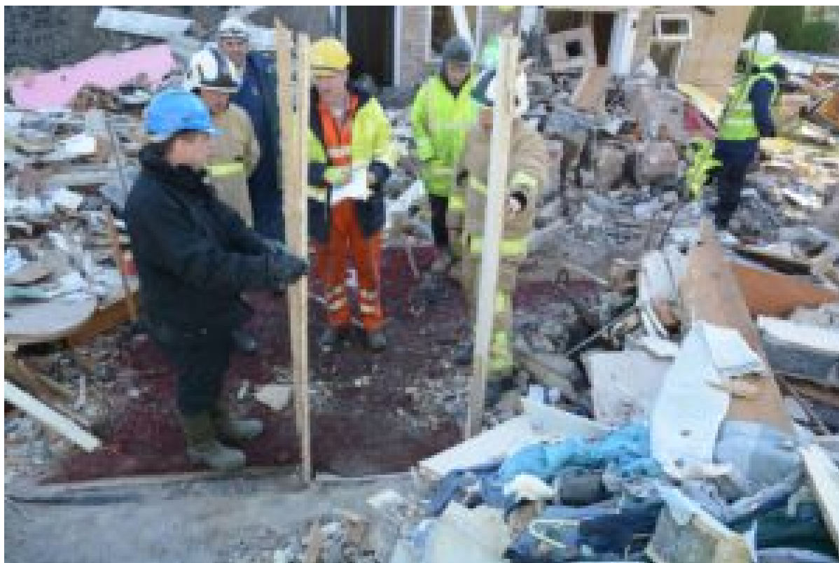
Steve attending the scene of a gas explosion in Haxby, York
