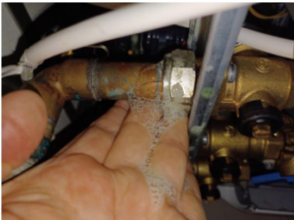
The leaking gas pipe
