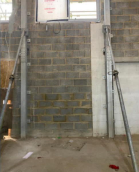
The door and the concrete ground below it
