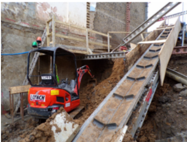
excavation and stability structure concerns
