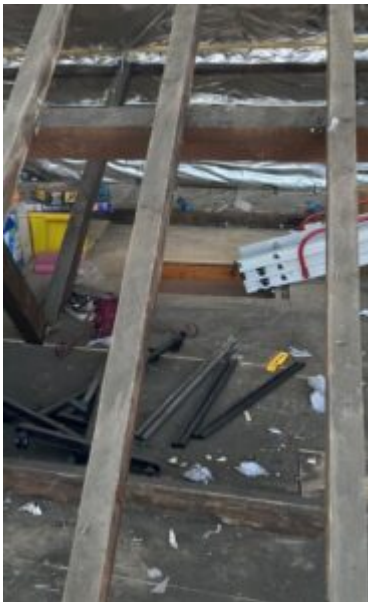
The unguarded loft hatch
