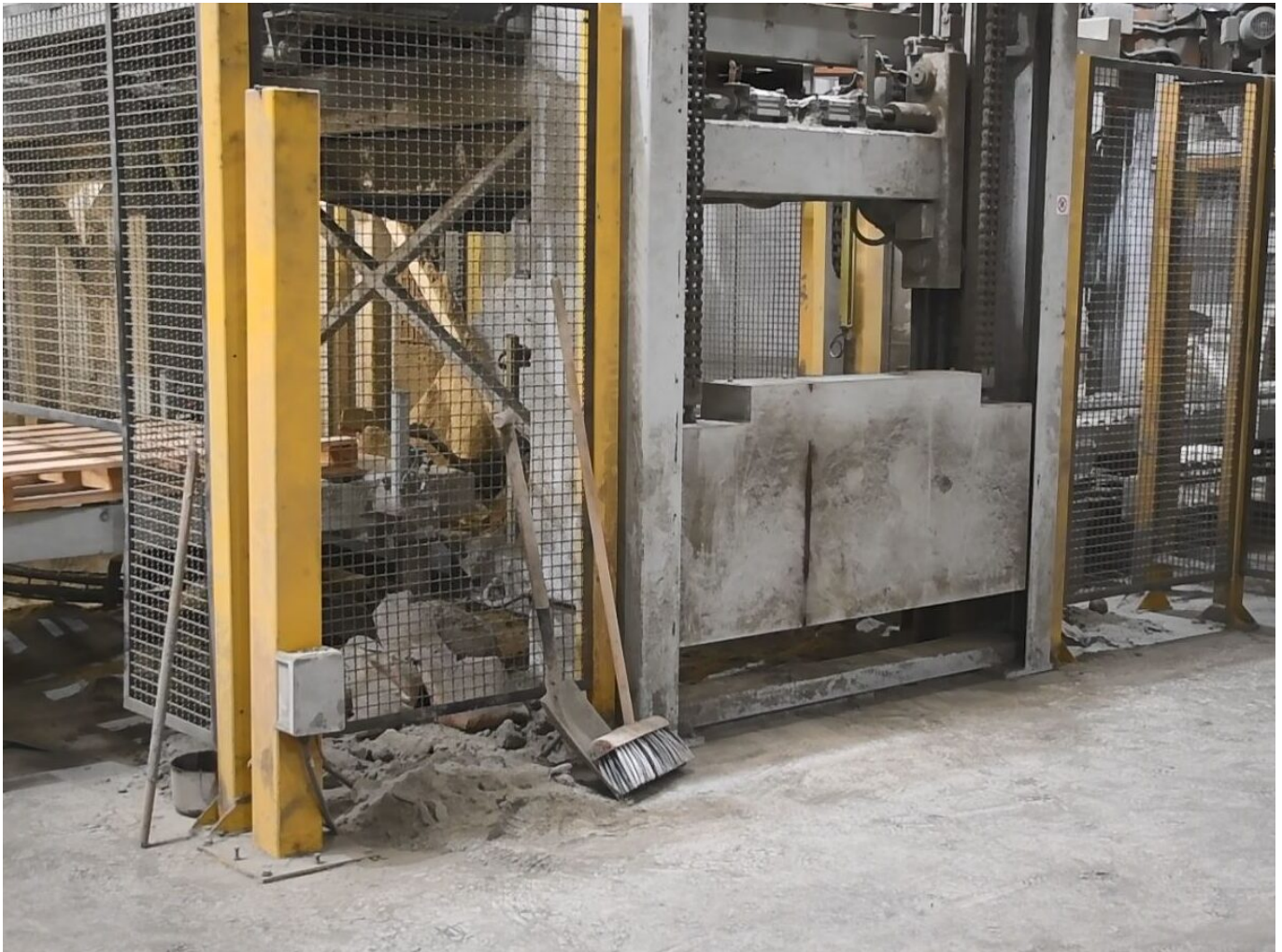
The unguarded concrete weight.
