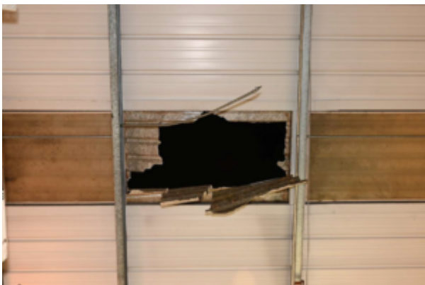
Broken roof skylight
