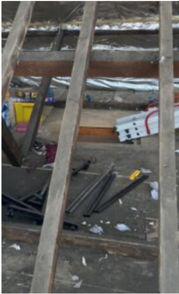
The unguarded loft hatch
