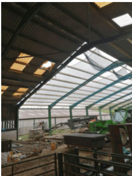
Jack Croft fell through the barn roof light
