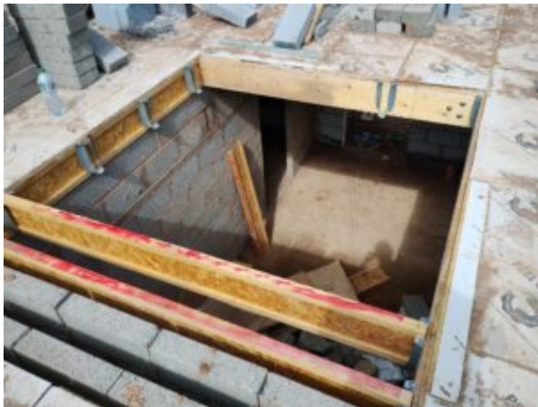
The collapsed stairwell after the incident
