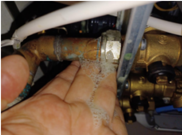
The leaking gas pipe
